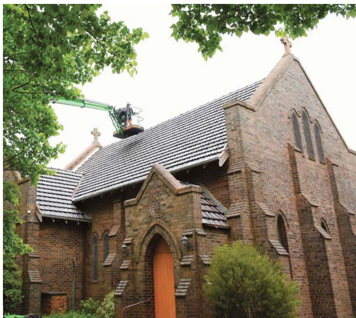
Contractor Steve Grant undertaking stage 2 work on the Anglican Church roof in 2018
