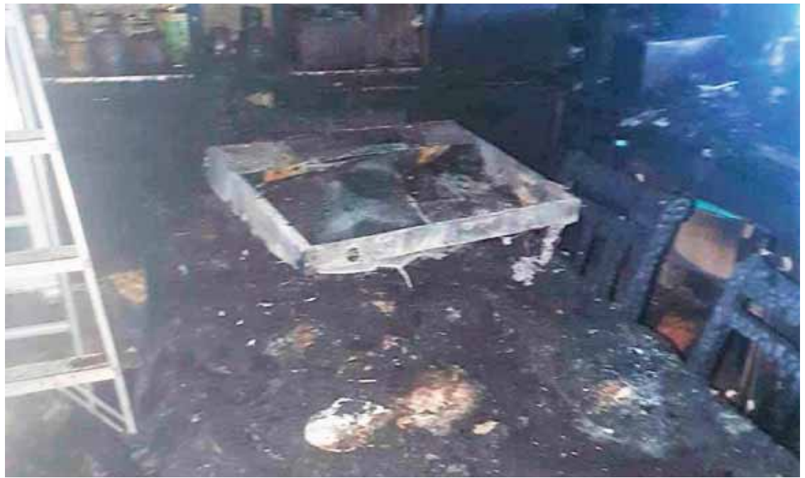
The Black Mountain home was extensively damaged in the fire
